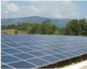
Solar Power Plant
